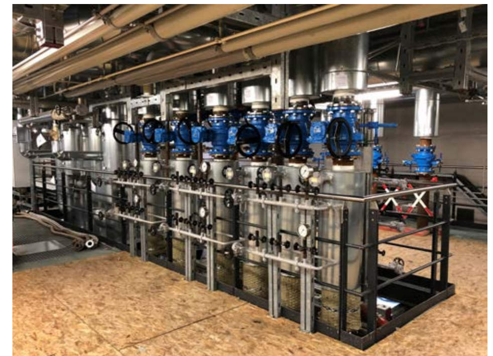
A row of DN 150 KLINGER Ballostar KHI ball valves installed at Erdwärme Grünwald
